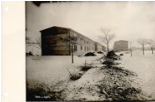
Halifax, N.S.: Apartments on South Common. "Roofing in" the last building on Endicott Avenue. (listed twice in the catalogue (68 & 71)
