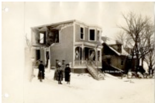
Halifax, N.S.: House. Showing apparently the outward force exerted by the explosion.
