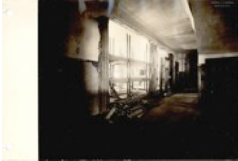
Halifax, N.S.: Interior of Alexander McKay School, showing the destructive force of the explosion.
