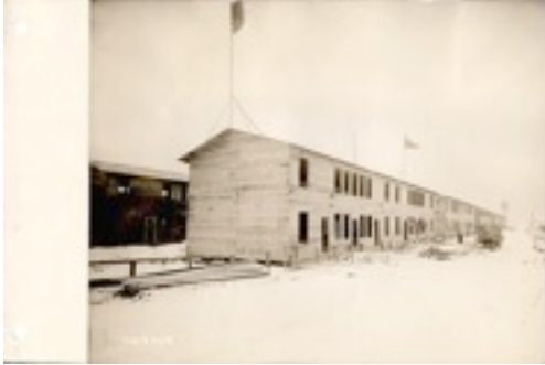
Halifax, N.S.: Last Apartment House of the Exhibition Grounds being "roofed in".
