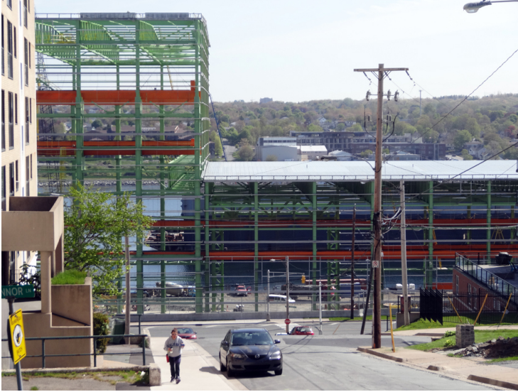
Irving Shipbuilding's massive fabrication shed, where Canada's new fleet of frigates and Arctic patrol vessels will be built, blocks the view of Halifax Harbour from a monument to victims of the 1917 explosion that killed almost 2,000. Dean Jobb
